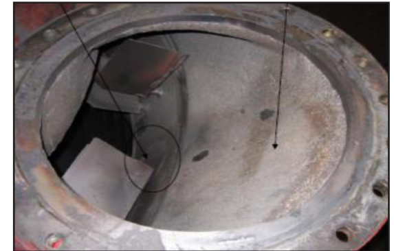
Outlet pipe after 40K hours showing small spots requiring repair with ARC
